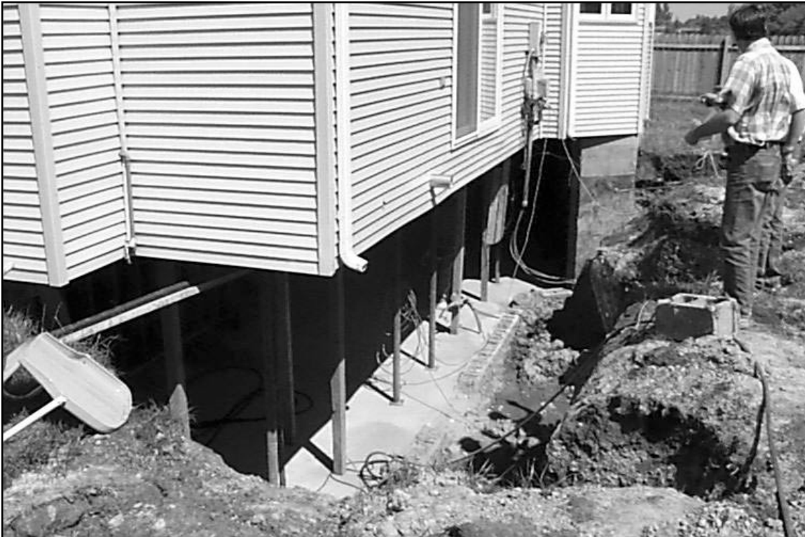
Figure 9 Failure of this unreinforced masonry basement during flooding in East Grand Forks, MN, in 1997 caused approximately $32,000 in damage.
